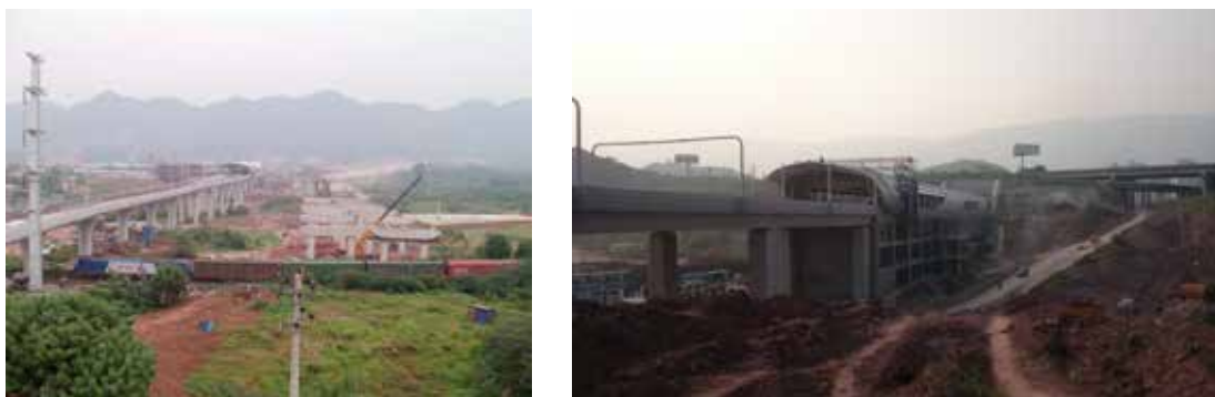
Figure 2: Monorail stations under construction in Chongqing (Left: Line 1, Laijiaqiao Station; Right: Line 6, Longfengxi Station)
